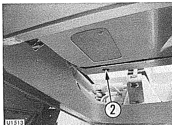
Drain valve (bottom of radiator)
